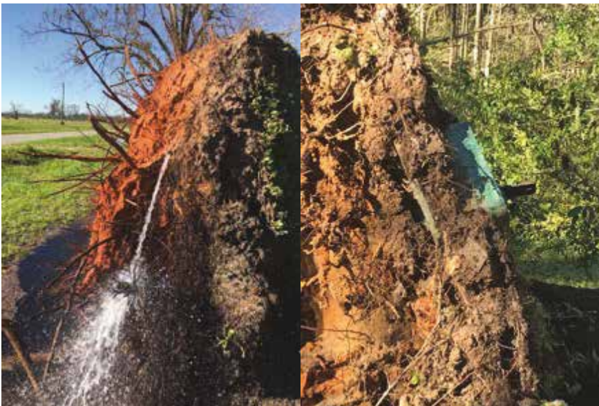
Pictured above: Water lines and water meter boxes that were "uprooted" when trees came down during Hurricane Michael
